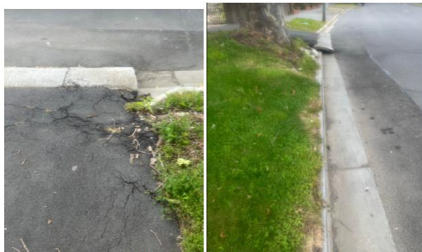
Good kerb/channel condition & minor driveway crossover damaged due to tree uplifting (27 Norwood Ave)
