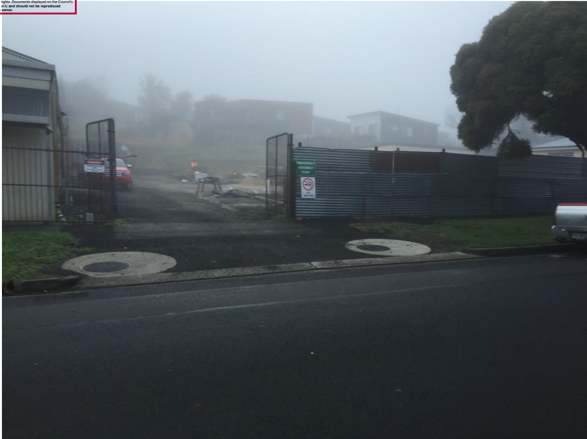
Fig 4.1a – View of new access under construction – upgrading to minimum 5.5m width required in progress
