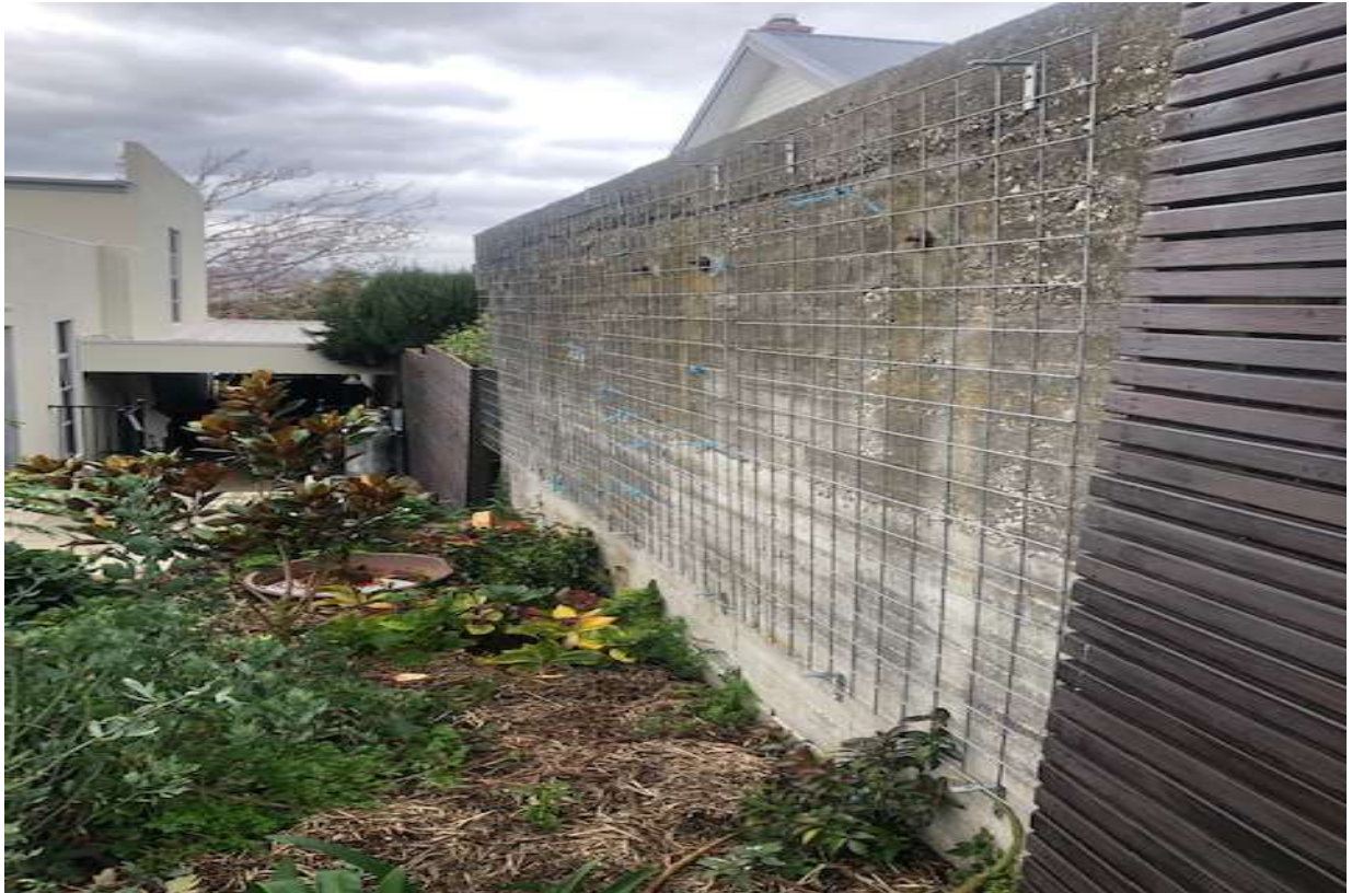
Figure 6 Section D-E Toppling garage wall
