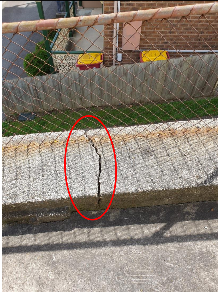
Large crack on top of bluestone retaining wall above staircase.
