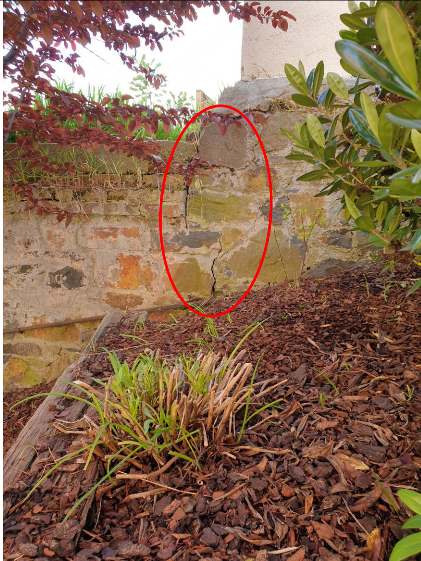
Southern house corner foundation crack
