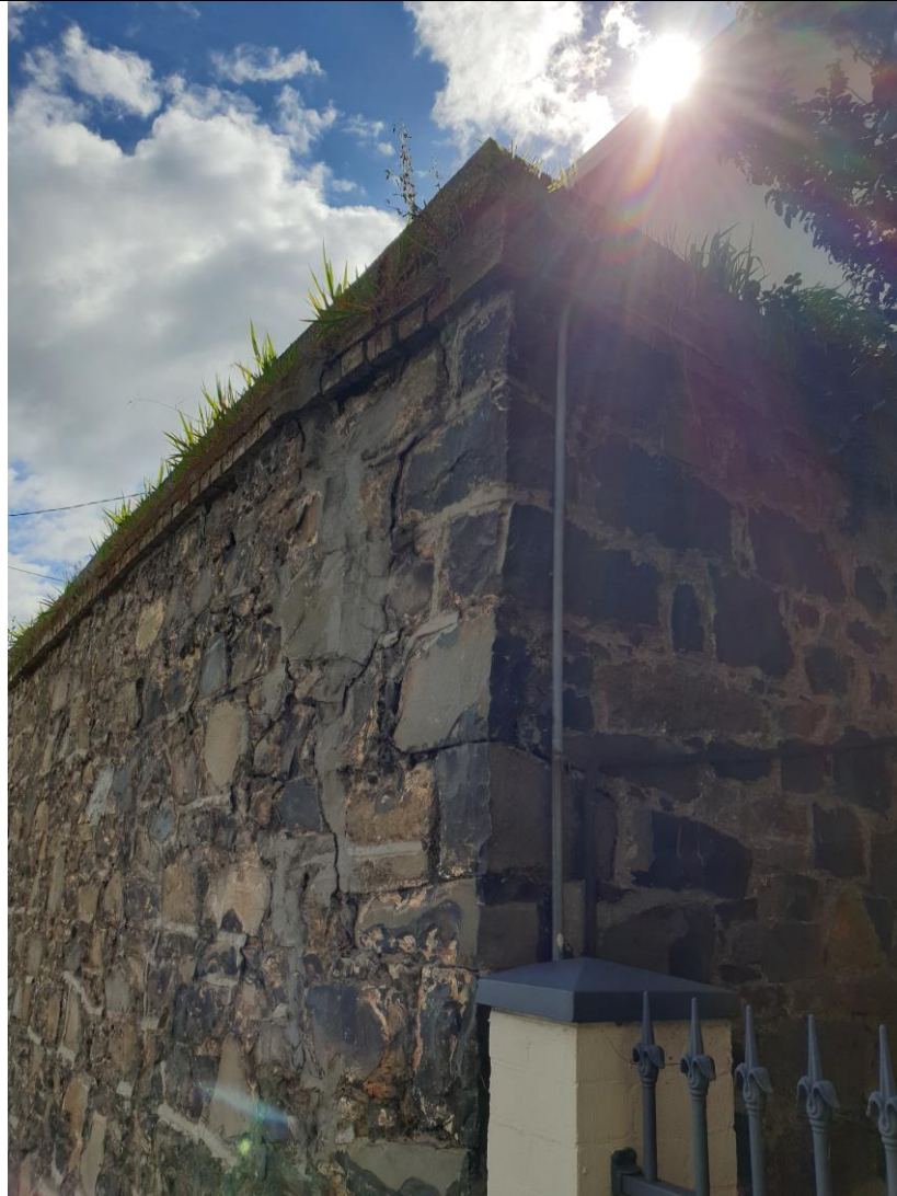
Cracking in southern corner of existing bluestone retaining wall Photo 2.
