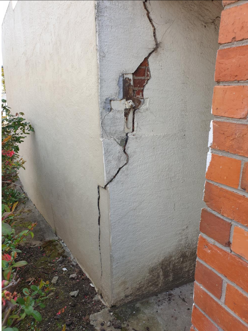
Southern house corner severe cracking
