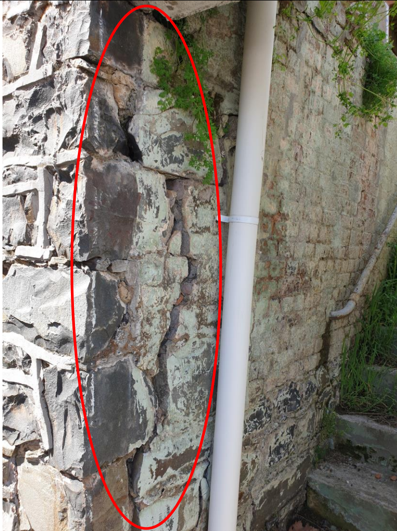
Large crack on within of brick/bluestone retaining wall adjoining the stairwell.
