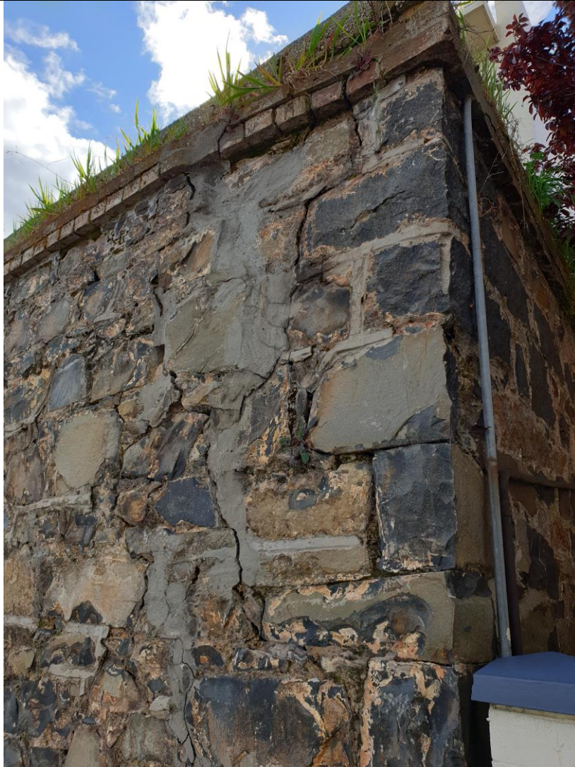
Cracking in southern corner of existing bluestone retaining wall Photo 1.
