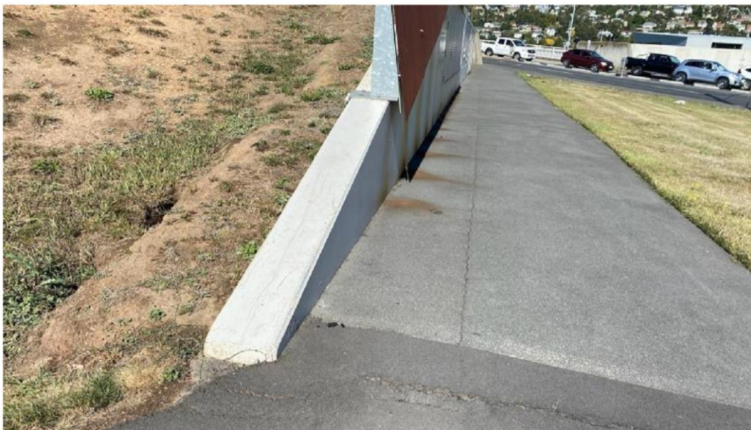
Invermay Levee (Goderich/Lindsay St.) - levee settlement at the earth/concrete interface
