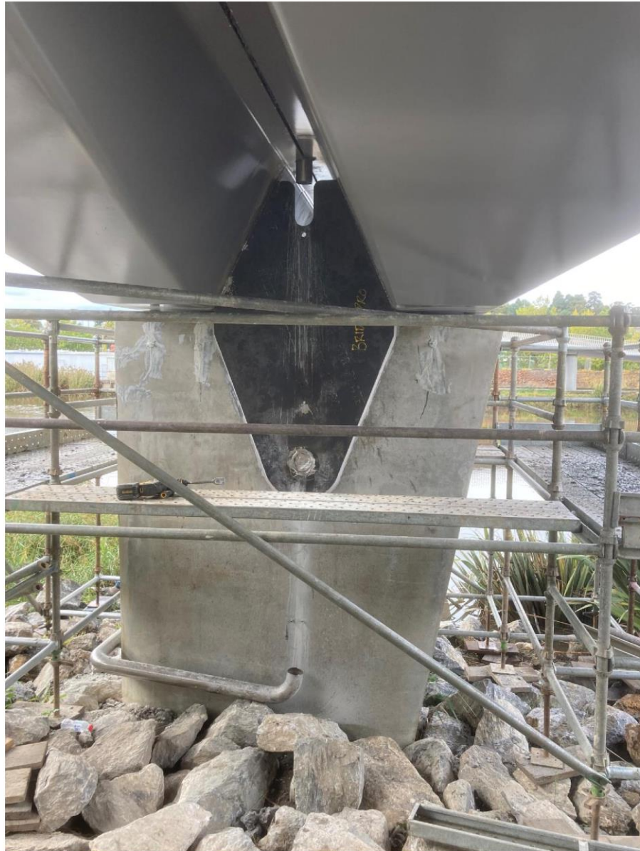
PHOTOGRAPH OF ADDITIONAL STEEL WEBPLATE AT TOP OF NORTHERN SIDE PYLON BEFORE CONCEALMENT BY CONCRETE CAPITAL AND 'BANDAGING' COATED OVER WITH APOXY-TYPE COATING
