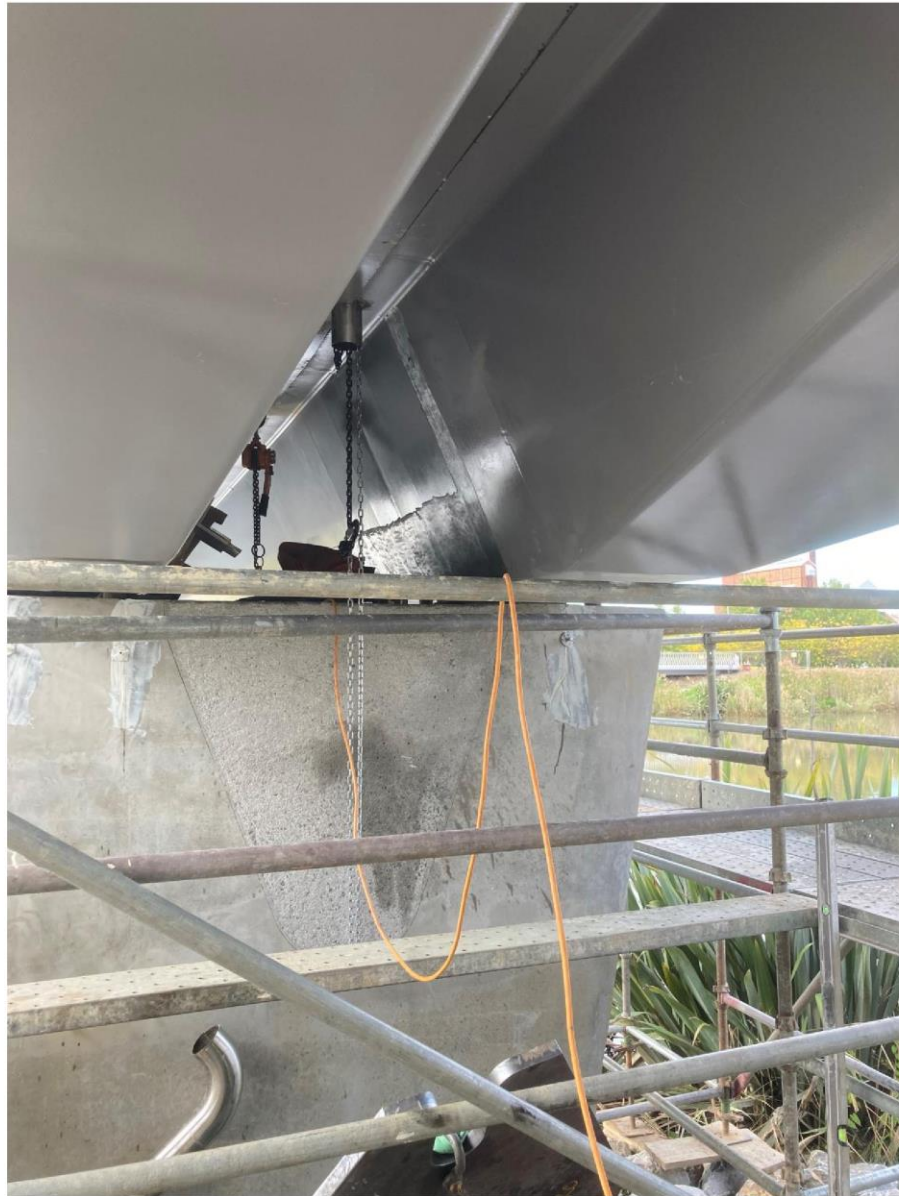
PHOTOGRAPH OF NORTERN PYLON SHOWING SEMI-PATCHED CRACKING, BEFORE INSTALLATION OF STEEL PLATE AND BEFORE 'BANDAGING AND COATING WITH EPOXY
