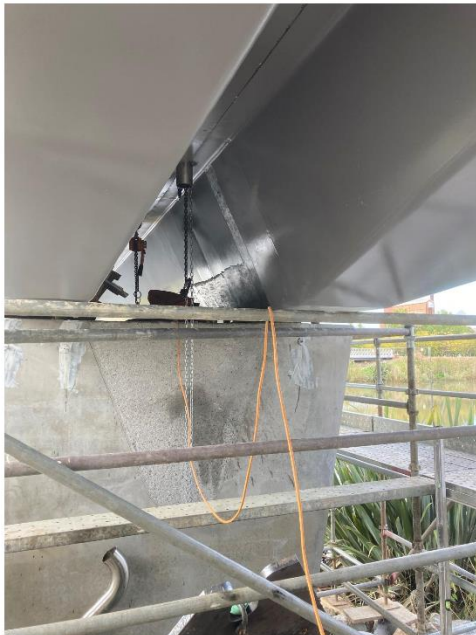
PHOTOGRAPH OF NORTHERN PYLON SHOWING SEMI-PATCHED CRACKING, BEFORE INSTALLATION OF STEEL PLATE AND BEFORE 'BANDAGING' AND COATING WITH EPOXY
