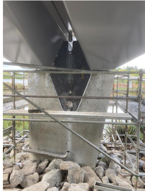
PHOTOGRAPH OF ADDITIONAL STEEL WEBPLATE AT TOP OF NORTHERN SIDE PYLON BEFORE CONCEALMENT BY CONCRETE CAPITAL AND 'BANDAGING' COATED OVER WITH EPOXY-TYPE COATING
