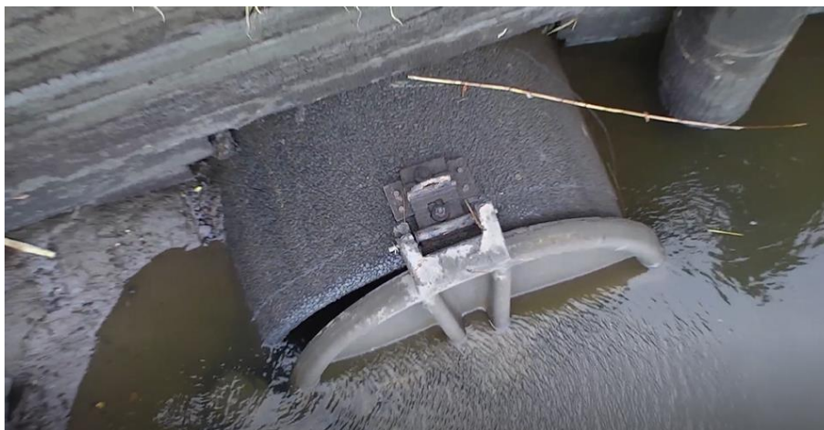
The broken tide flap identified with drone surveillance
