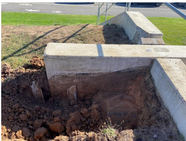
Buried buttress and sheet piling visible at the junction of the concrete wall and wing wall
