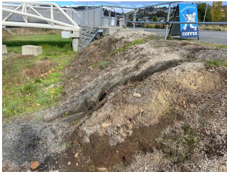
Site of Riverbend levee erosion before intervention
