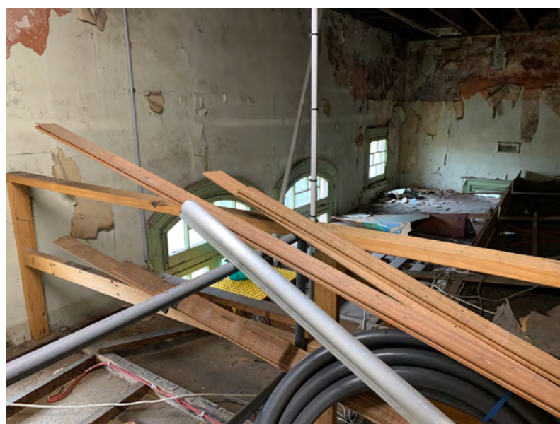
Projection room above the John Duncan Centre (JDC) created by lowering the JDC ceiling
