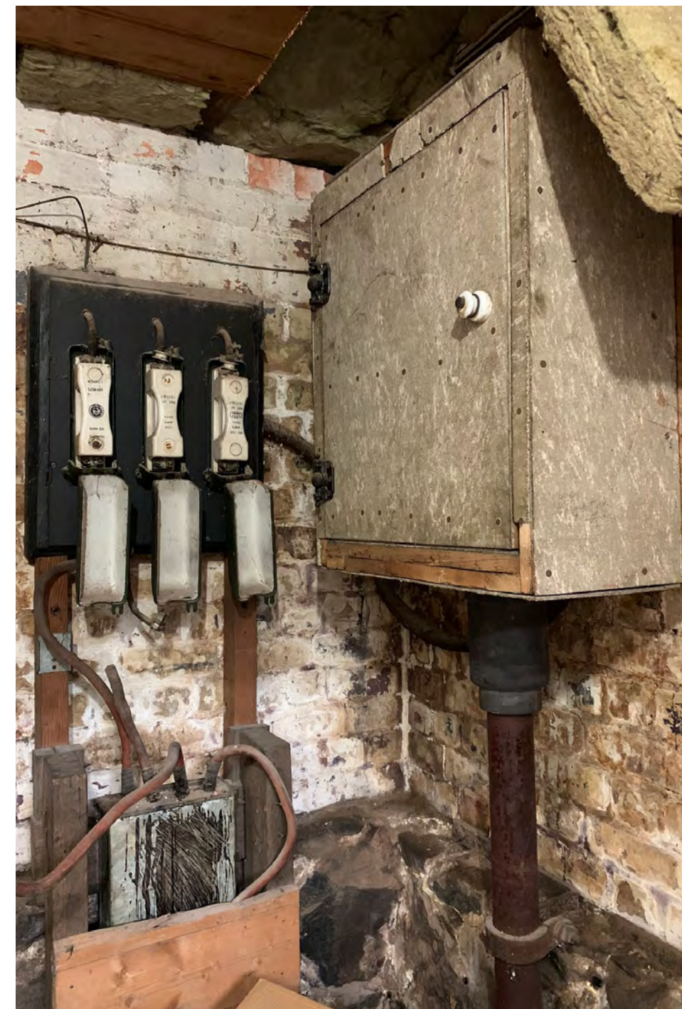
Basement original electrical switches for power from Duck Reach Power Station. Note asbestos containing casing to power board.
