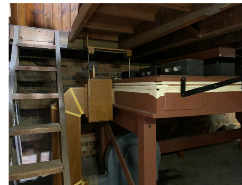
The Organ's electric blower (to supplement the hydraulic engine), kangaroo skin-lined horizontal bellows and ladder up to the Organ Chamber.
